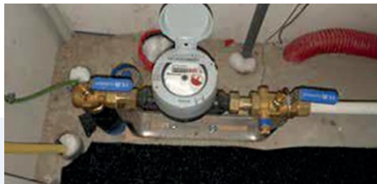
Waterleiding is open
