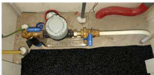
Waterleiding is afgesloten Water Supply closed
